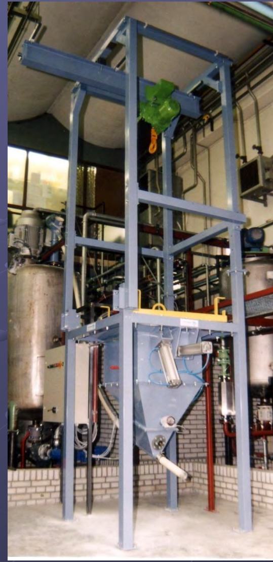
← ↑ Loading of the station using a crane runway which is integrated within the emptying station
